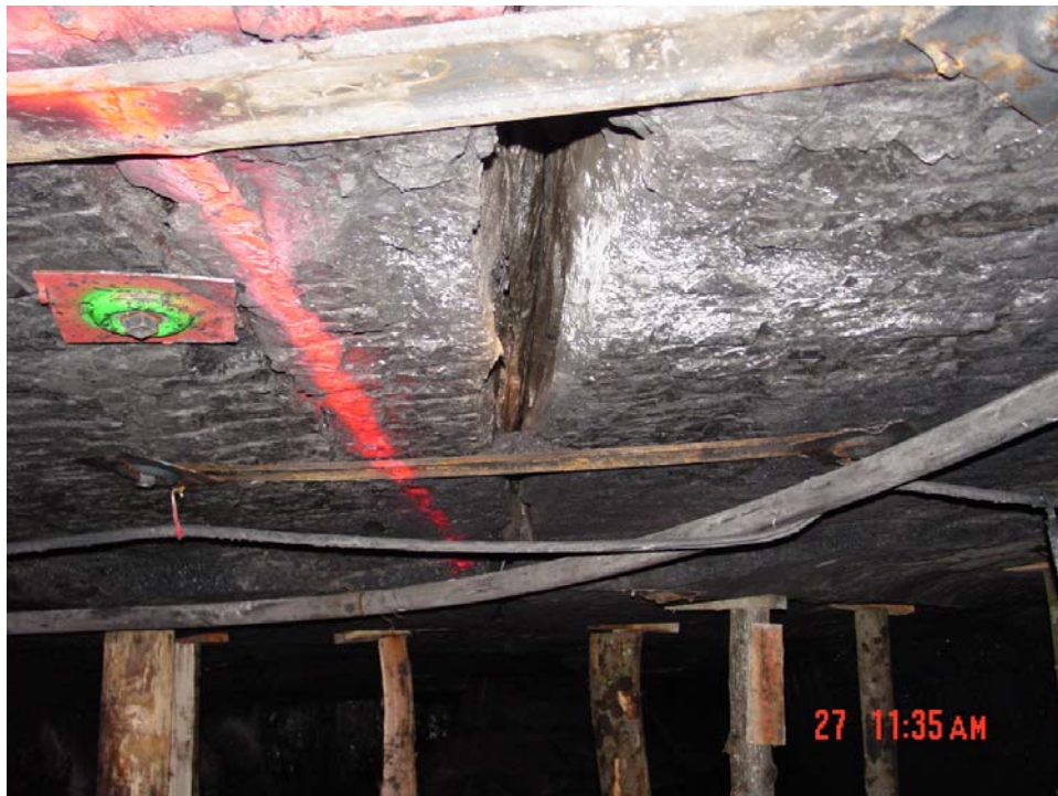
Figure 5. Open Joint in Mine Roof
