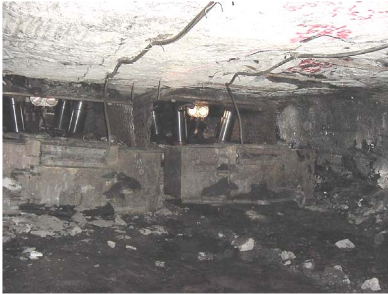
Figure 3. Mobile Roof Supports on a Retreat Mining Section
